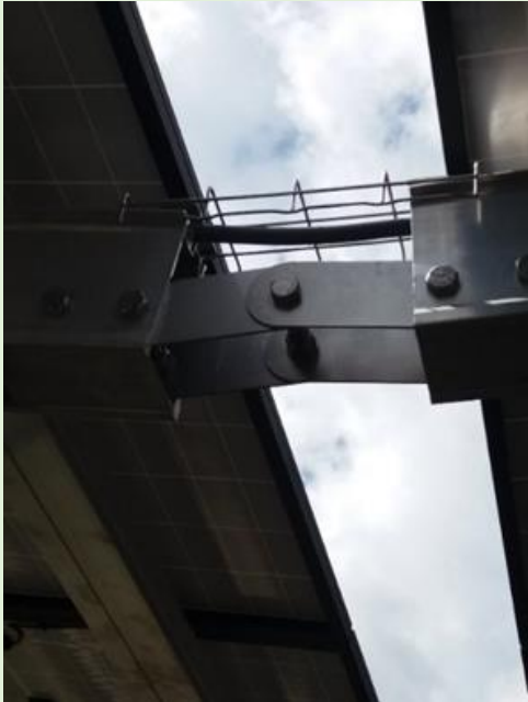
Protection of cables against flying objects or collapsing structures (Carport at Union, Saint Lucia)
